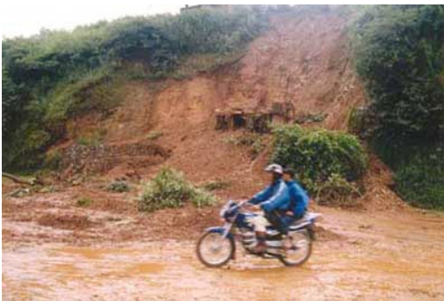
Figure 6. Flow-like landslide on roadside slopes of southern hills of Kathmandu, triggered by Rainfall of July 2002
