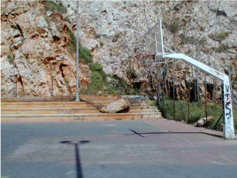
Figure 10. A big rock mass block coming from the fractured and karstificated zone mentioned in Figure 7. It caused damage on the tiers and on the fence of the basket ball field.
