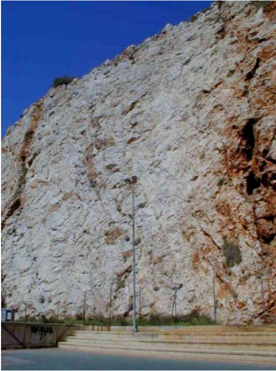
Figure 9. The basket ball field including the rows of seats are installed on the base of a slope (30m high), without keeping any safety distance. The section of the slope presented in this figure is intersected by a fractured and karstified zone filled with stalagmitic materials.
