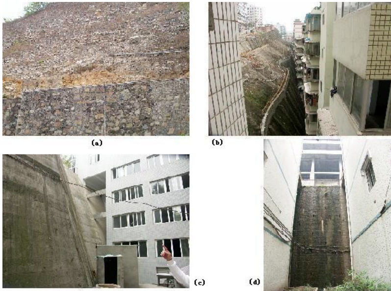
Figure 4. Problems in slope reinforcement
