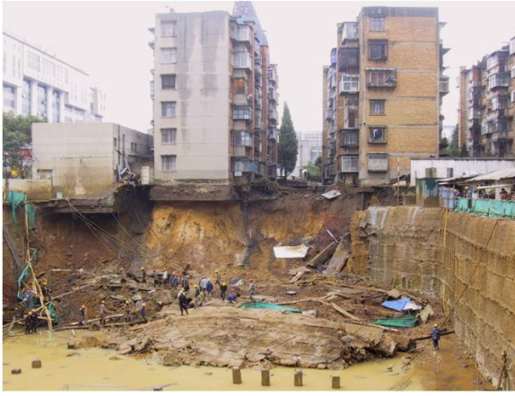
Figure 8. Slope failure of foundation pit A in Kunming city
