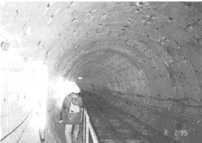
Figure 6. Post Earthquake Inspection of the Isobe Dori Shield Tunnel, Kobe, Japan Source: JSCE, 1995
