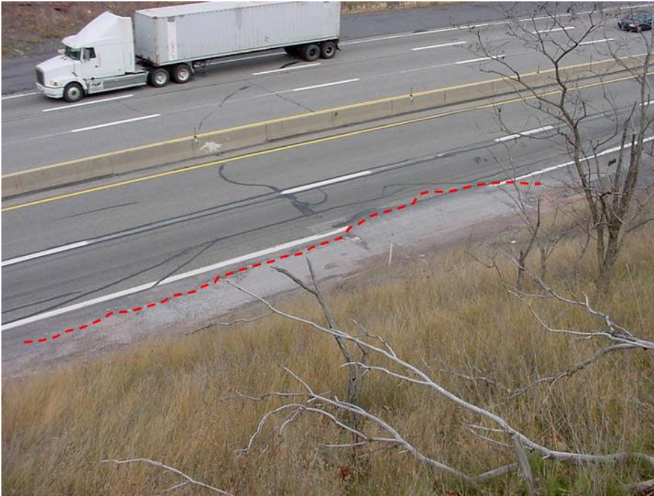
Figure 3. An overview of pavement heaving of eastbound lane of I-76.
