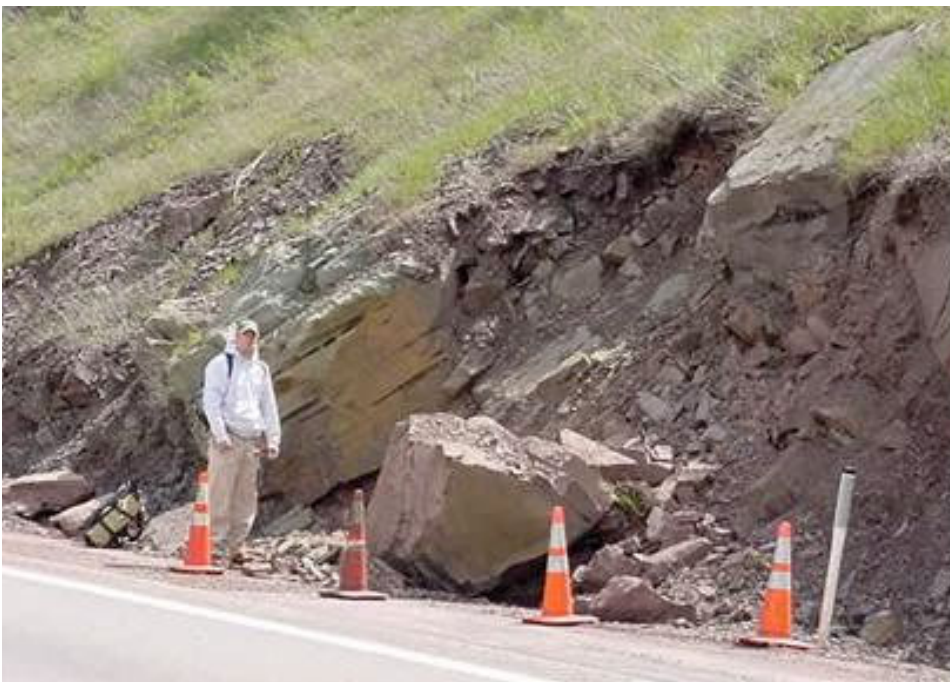
Figure 4. A major rockfall within the toe area of New Baltimore Landslide along I-76 in July of 2001.
