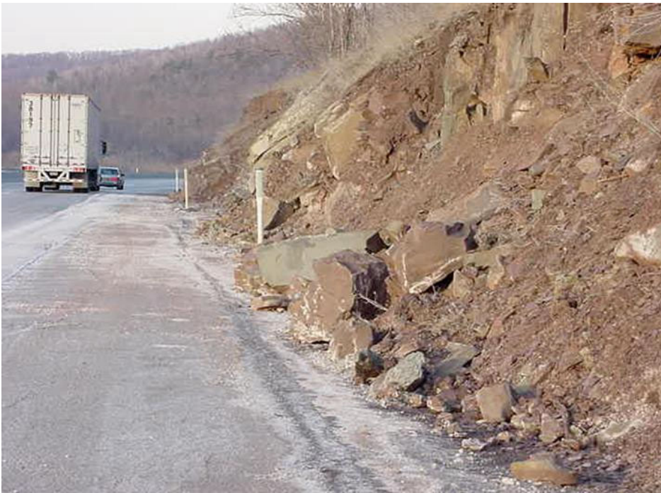
Figure 2. Overview of unstable rock mass at the toe of the landslide along I-76.
