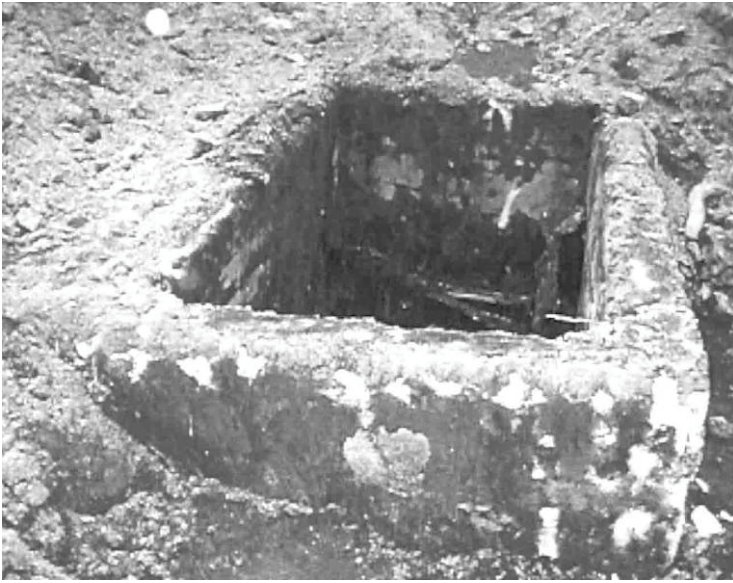
Figure 3. Concrete tar separator box discovered during site remediation at Dover, New Hampshire. The box measures about 2 x 3 m in plan (Courtesy of New Hampshire Department of Health Services, Concord, N.H., 2002)
