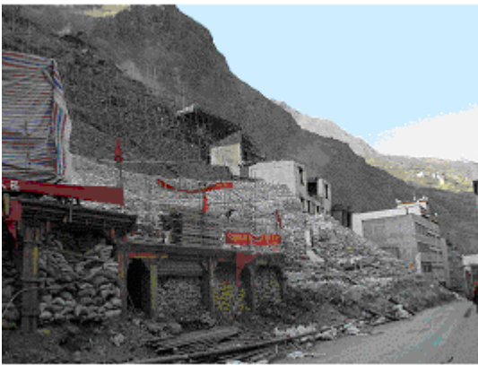
Figure 6. The sand bags piling engineering in the leading edge of the landslide
