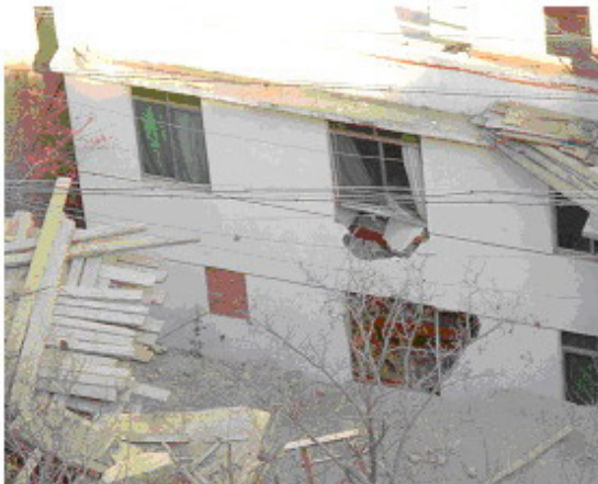
Figure 5. The houses destroyed by the partial slumps in Region II at the foot of the landslide
