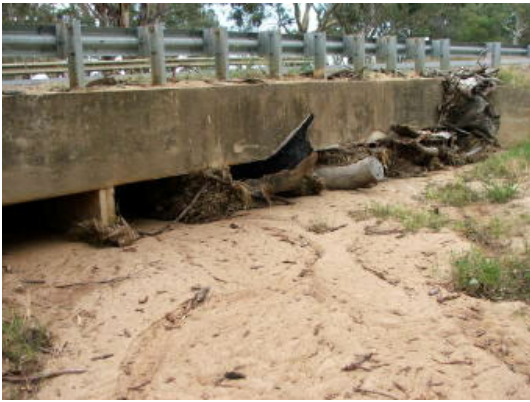
Figure 4. Sediment impact on bridge and road infrastructure
