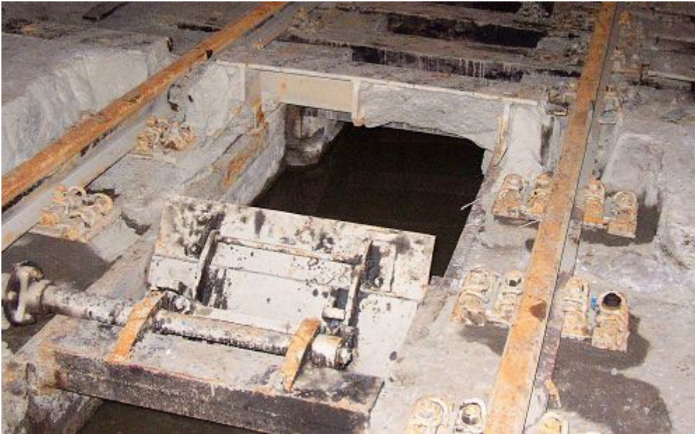
Figure 12. Pulled out concrete block in pressure divide
