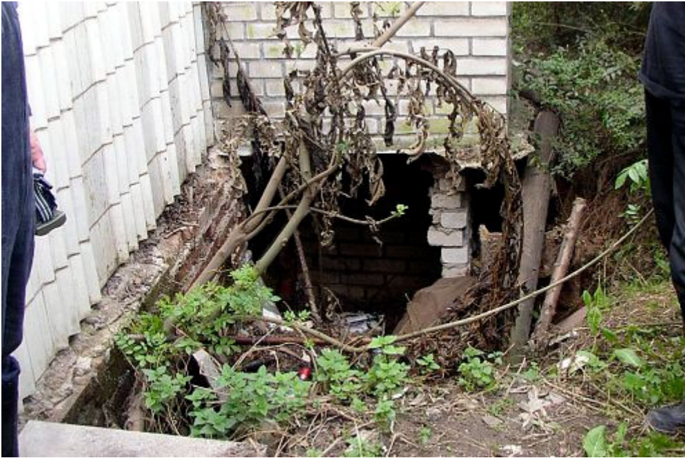
Figure 10. Damaged ventilation shaft near Invalidovna Station
