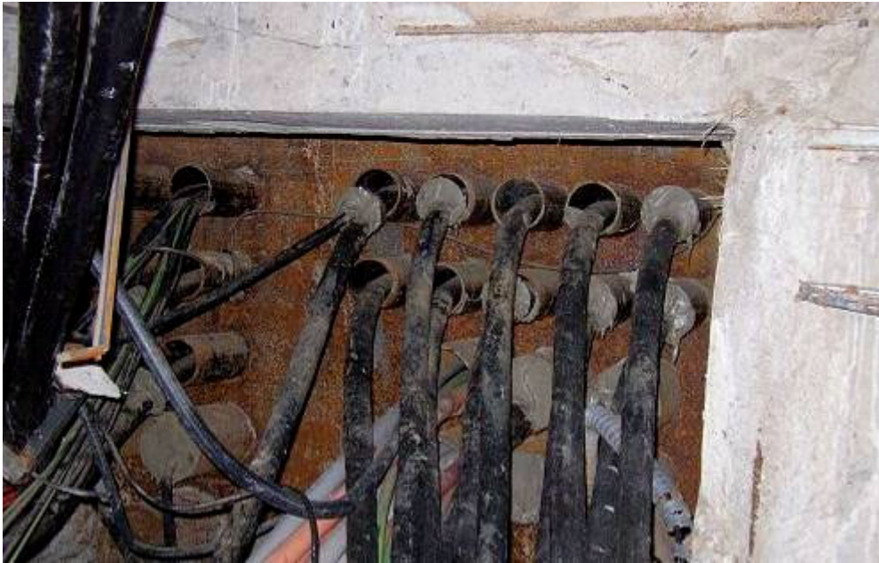
Figure 14. Unsealed cable grommets
