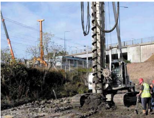
Figure 11. CFA piling operation (foreground), in lieu of vcc's within proximity to existing drain, on alignment of motorway embankment widening approach to location of new bridge crossing over metro-link tram line and Bridgewater canal. Existing M60 motorway bridge in back ground.
