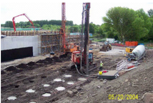
Figure 3a. Vibro concrete column (vcc) installation for embankment approach to piled bridge abutment.
