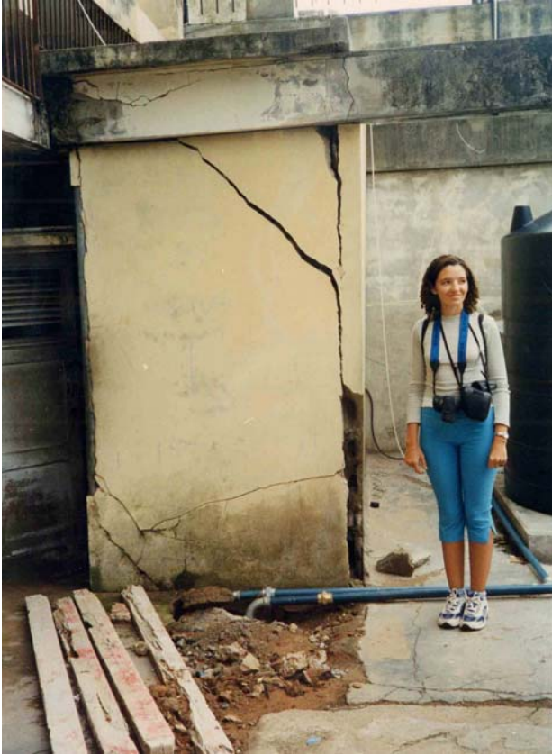
Figure 5. Site 1, damage to a single story construction on the left hand side at the back of the building.
