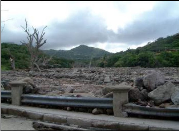
Figure 5. The Belham Valley Bridge with lahar deposits up to deck level. The lahar deposits consist of granular, variable, well-rounded, highly spherical, cobbles & boulders (mainly andesite and dacite) and sub-rounded, elongate cobbles and boulders with preferential alignment and cross laminations. The deposits were loosely packed, highly permeable, porous, saturated, with occasional clay and silt, some rootlets and tree stumps. The bridge deck currently lies at least 3.8 m below existing ground level.
