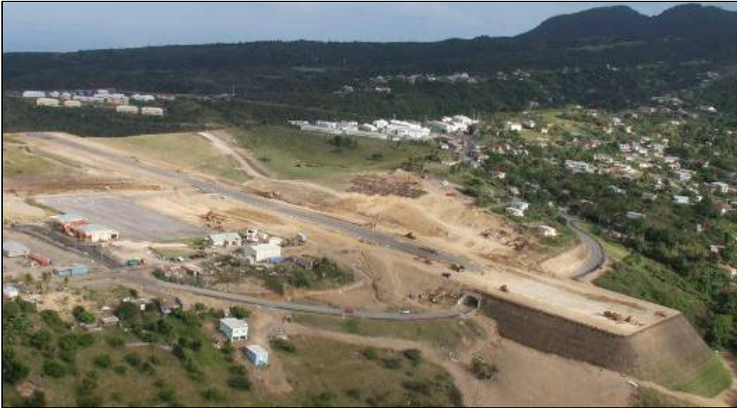
Figure 6. Photograph showing Gerald's Airport and the reinforced earth slope at the west end of the airport runway.
