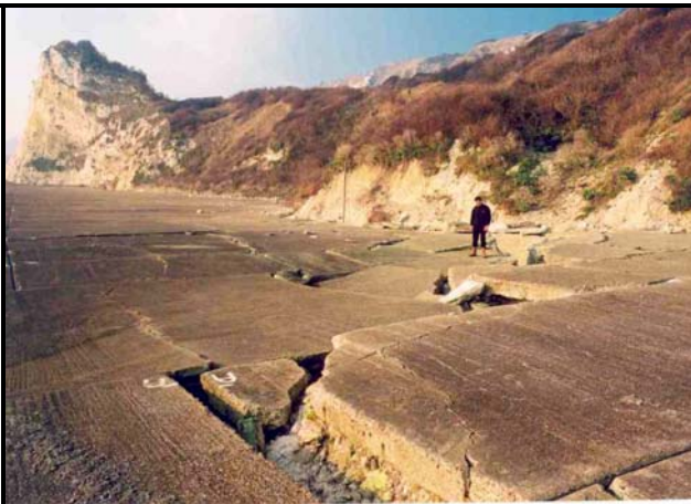
Figure 9. Severed concrete apron at Horesehead Point in 2001.
