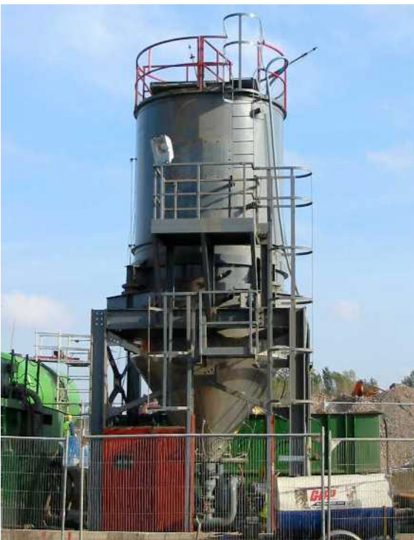
Figure 10. Bioreactor at Garston Gasworks
