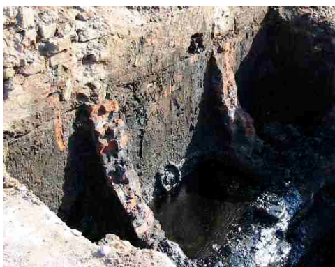
Figure 4. Free tar within a subsurface tar collection or storage tank
