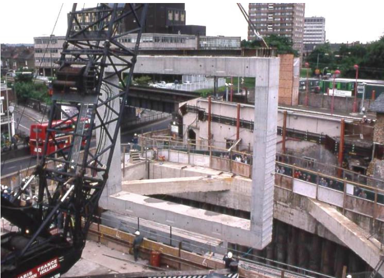
Figure 8. Lifting tunnel segment into jacking pit with railway station and bridge in background
