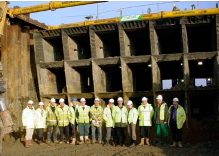
Figure 10. Cellular shield with steel plated cutting edges exposed at end of tunnelling
